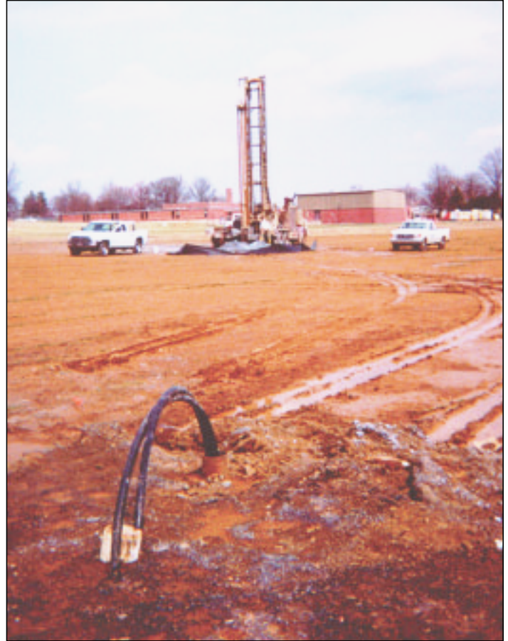
"Installation of wells and loop piping for ground source heat pump system and geothermal test."
