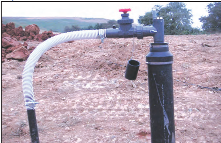
Landfill Gas Well
